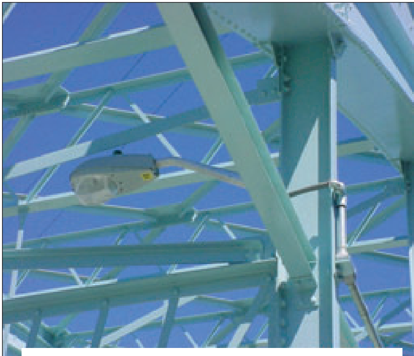
Lights were evenly spaced across the main span and were mounted higher and directly to the hangers.
