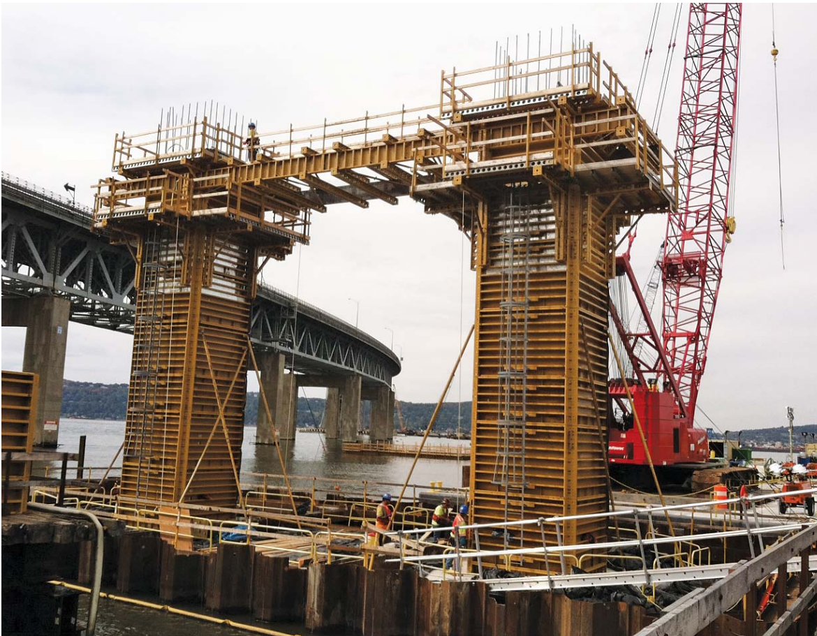
Two of the New NY Bridge's 136 pillars rise out of the river.
