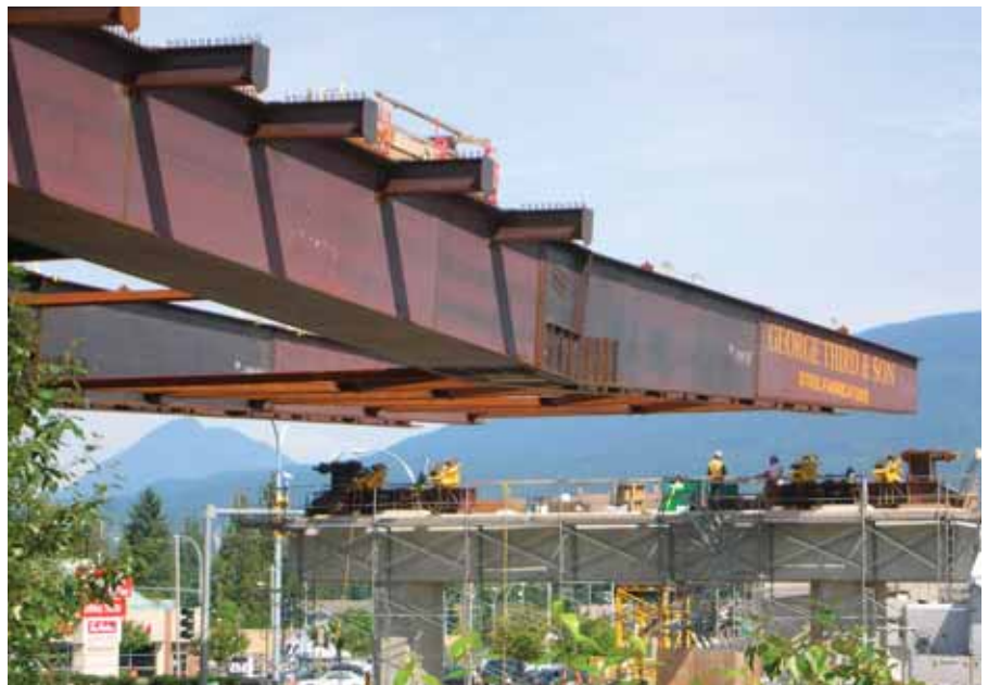
During launching the leading cantilever span required supplemental temporary stay-cable supports. The back spans had smaller demands. The 10-ft-deep box-girder sections alone were adequate for the trailing spans during launching.
