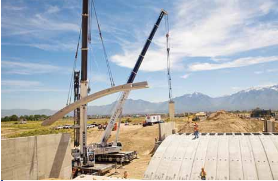
It took only two days to set the 20 precast arches; each arch was formed by two 4-ft-wide, 42-ft-long, 2-ft-thick precast units that joined together in the midspan.
