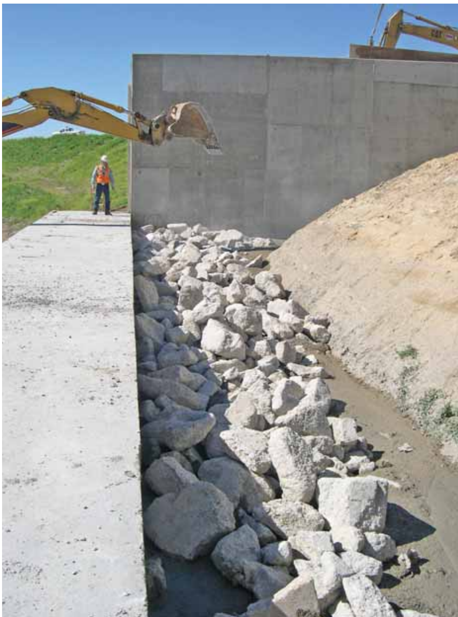
In an effort to save costs, fulfill Kennecott’s commitment to sustainable development at Daybreak, increase strength and shorten the time to place flowable fill material, the Daybreak/Nolte team used the 4,000-psi concrete slab waste material to help fill some of the void/area where the flowable fill thrust blocks were to be placed.
