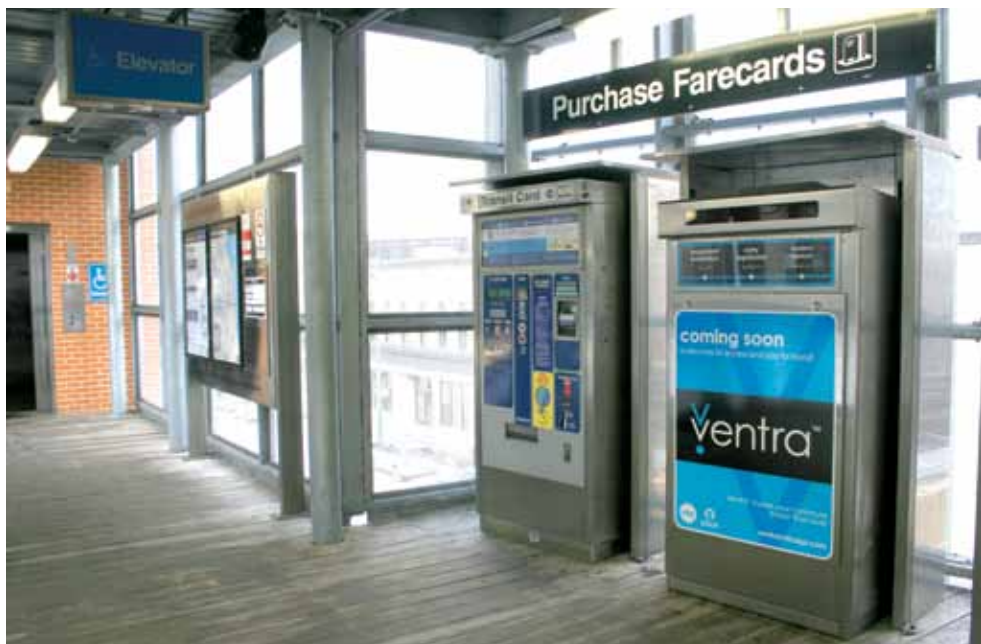
One of the biggest steps in implementing open payments is upgrading the infrastructure to accept open transactions at the point of service, such as metro gates and buses.
